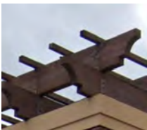
8 WOOD PERGOLA BROWN TEAK WOOD REF. MATCH EXISTING SHIPPING CENTER REF. COLOR CUSTOM BROWN SEE 3/A-400
